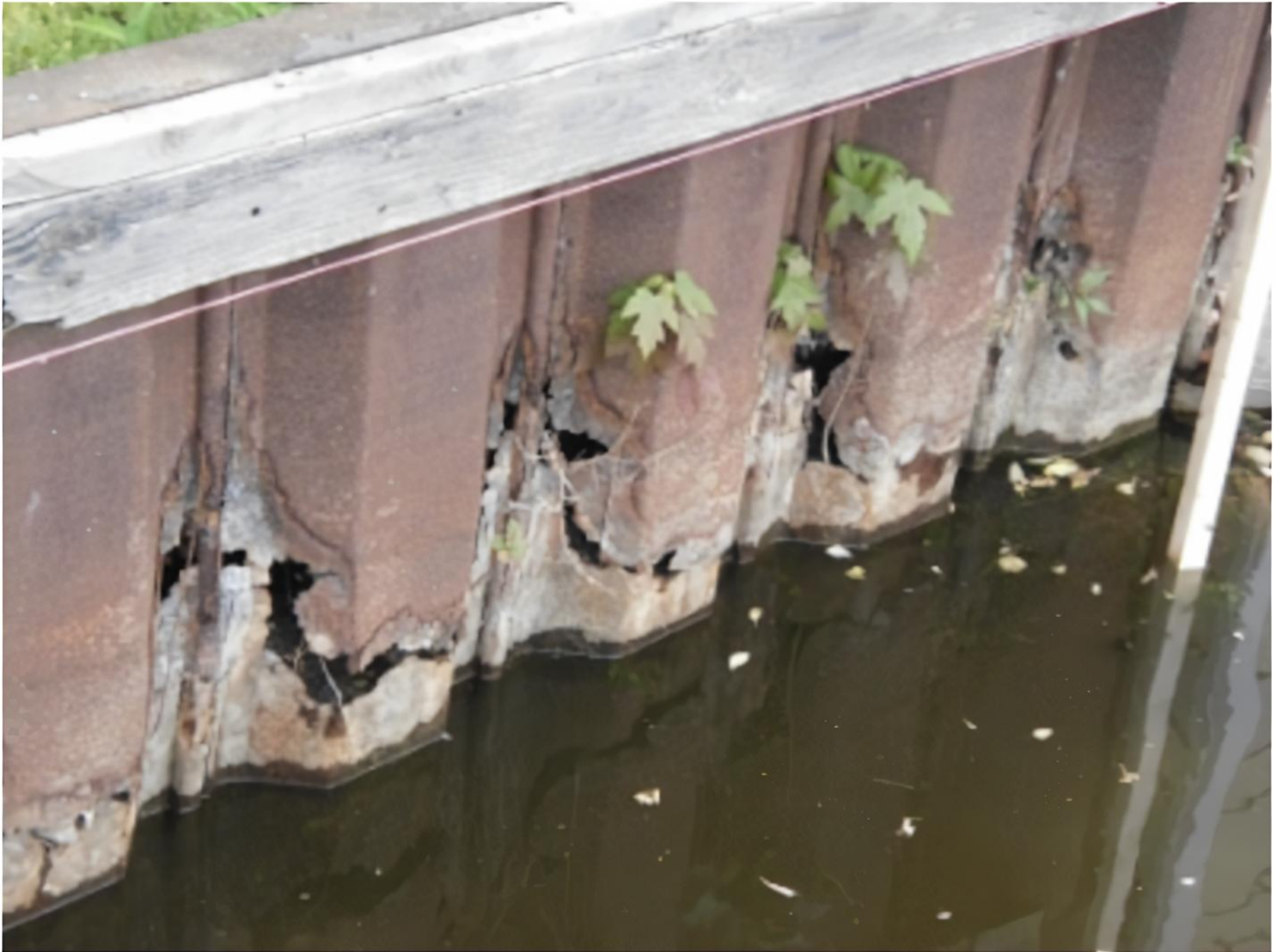
A photo of the defendant's retaining wall (Taken October 15, 2023)
